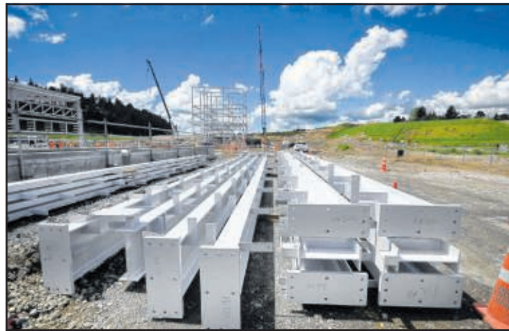
PERFORMING WELL: Massive new $400m Winstone Wallboards plant rising in the Bay of Plenty. NZ Herald picture
